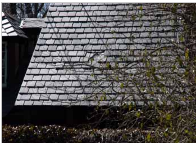
Figure 47. Slate roof in Phillips Mill residence. Although a few slates in the center have been broken by mechanical damage (probably a tree limb), replacement of the broken slates is readily accomplished without disturbing surrounding slates.
