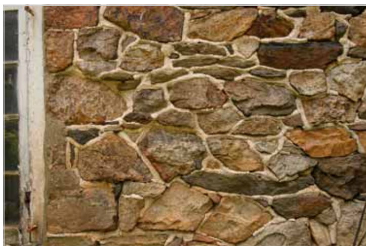
Figure 32. Detail of eighteenth century pointing. The most common joint profile type for rubble stone masonry was the raised ridge joint.
