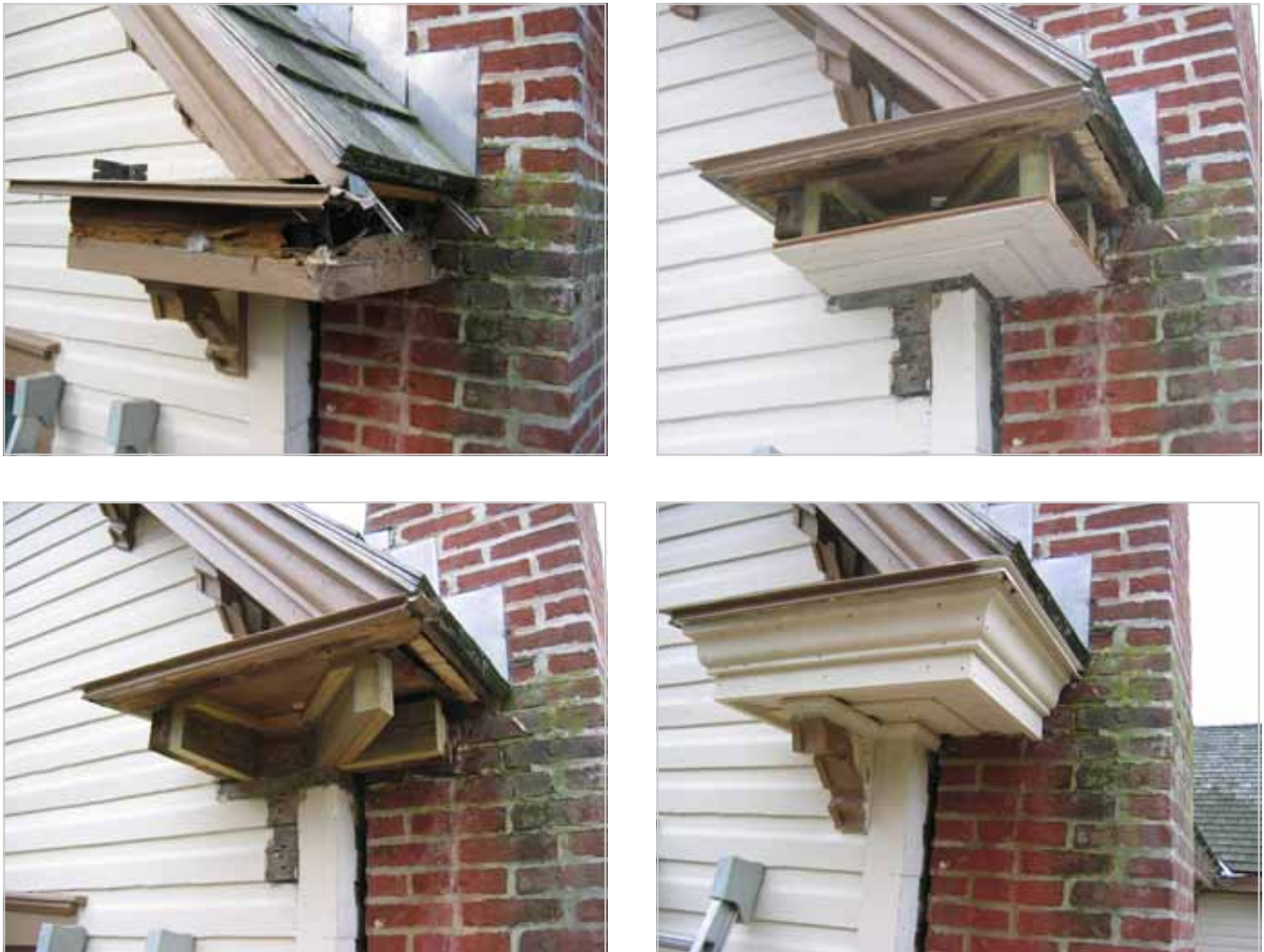
Figure 24. Sequence of restoration of a severely deteriorated cornice return. The crown molding was custom-cut for the project, a procedure that requires scheduling but does not add significantly to the repair cost.
