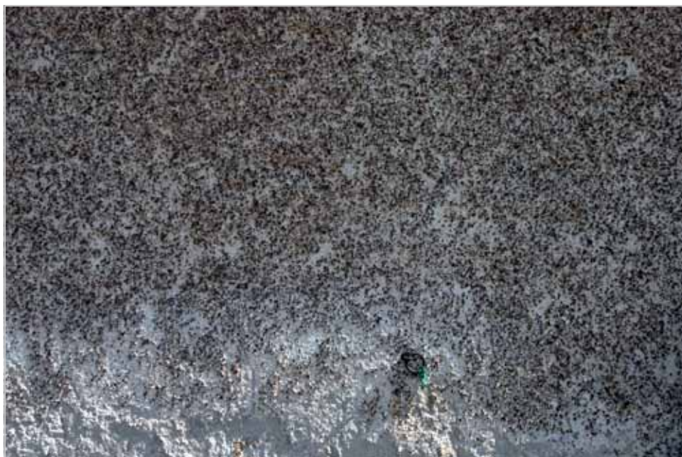
Figure 53. Detail of historic pebble-dash stucco, store building, Carversville Historic District. Surviving historic pebble-dash stucco is not commonly encountered.
