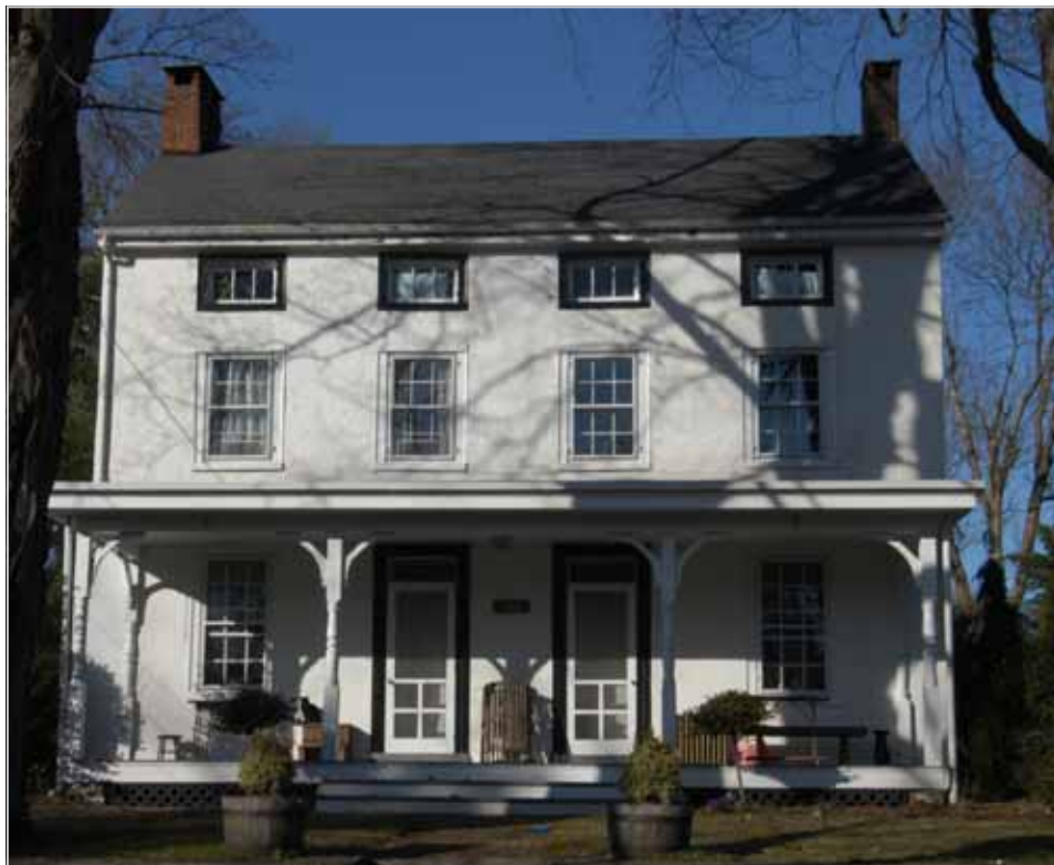
Figure 37. Preserved historic porch on Thomas Carver House, Aquetong Road, Carversville Historic District. Note the wood-framed porch and porch deck, wood steps, stone walks and steps, stone retaining walls, and stone sidewalk.
