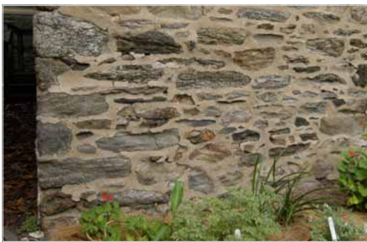
Figure 33. Overly-hard Portland cement mortar restrains the expansion of permeable stone masonry and results in the delamination (loss) of the face of the stone.
