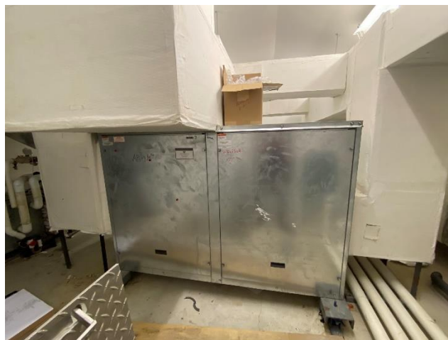
Energy Recovery Ventilator ERV-2
