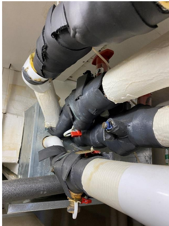
Insulation on Chilled and Hot Water Valves
