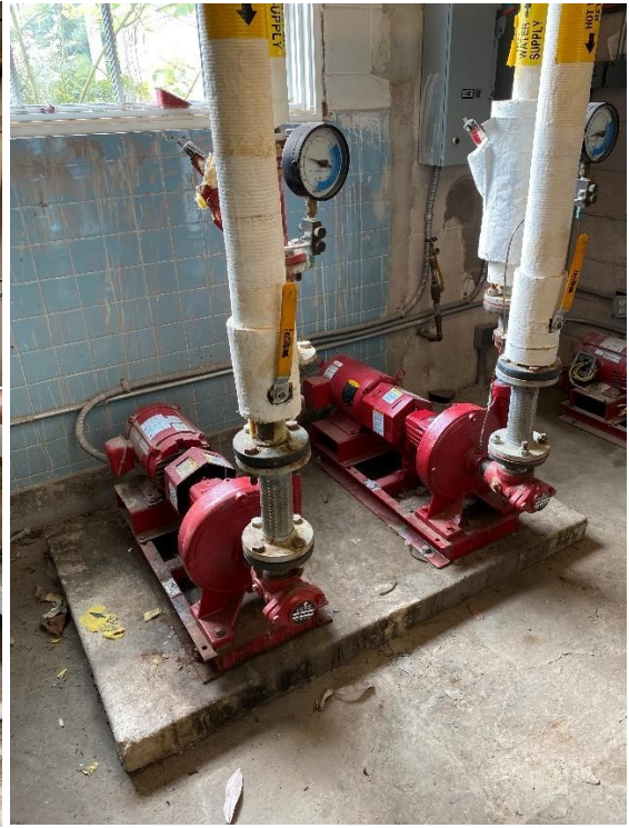
Hot Water System Pumps
