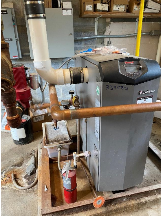
Hot Water Boiler
