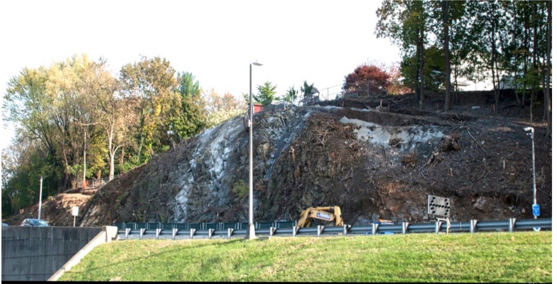
Actual After Defoliation Scaling RT 22 Phillipsburg Area Fall 2021 Photo
